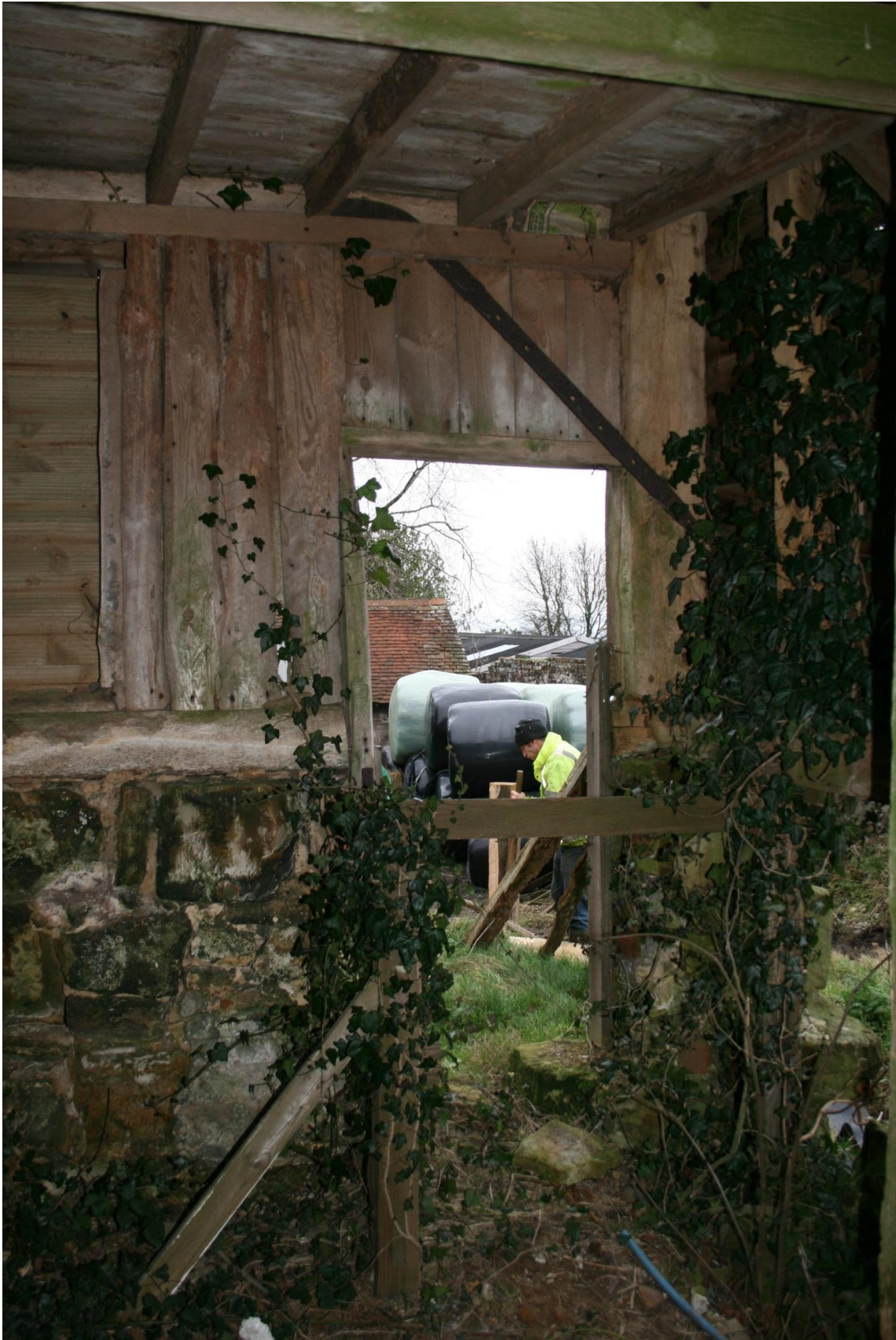
Plate 33 Before renovating inside looking through north east corner doorway (Reproduced by kind permission of Jamie French)
