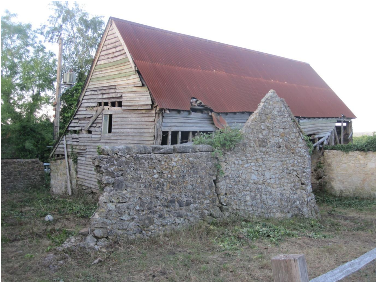
Plate 34 Before renovating looking towards the south elevation (Reproduced by kind permission of Jamie French)
