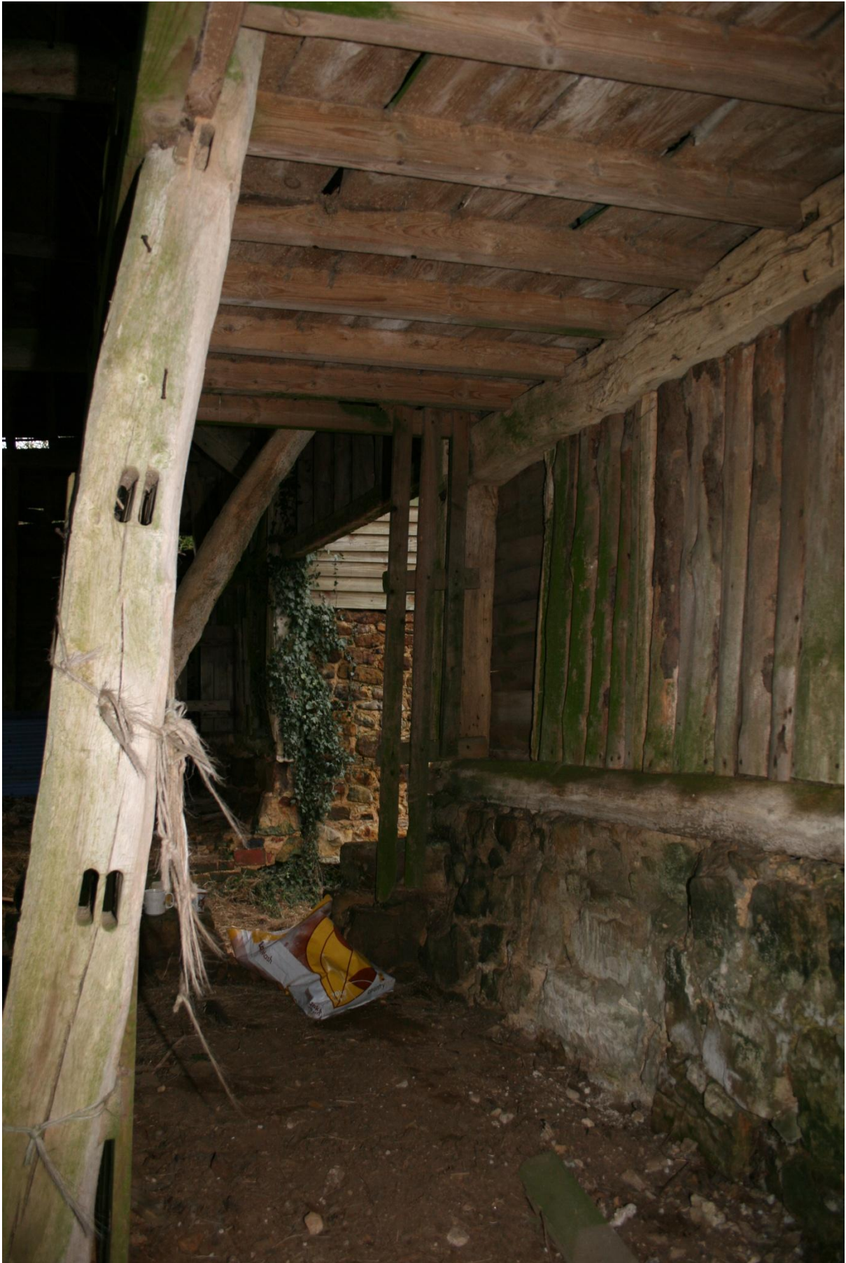
Plate 32 Before renovating inside looking north west from far side (Reproduced by kind permission of Jamie French)
