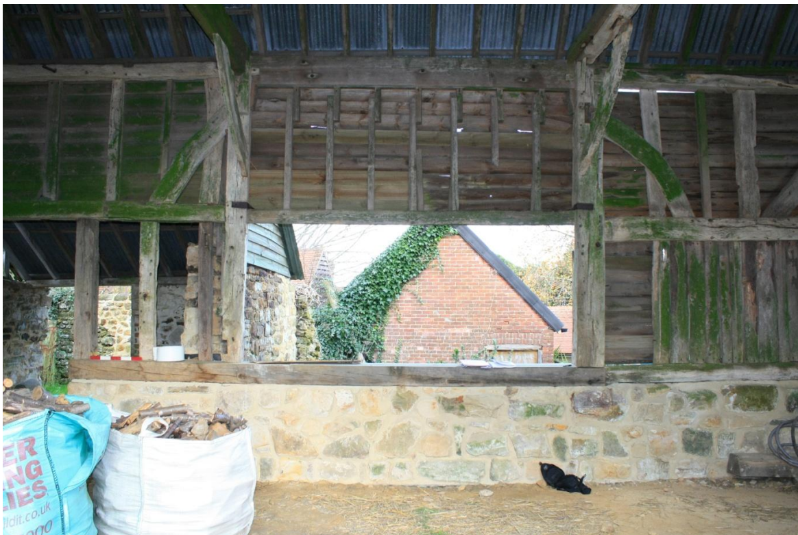
Plate 17 Half height entrance with new plinth built between truss B and C
