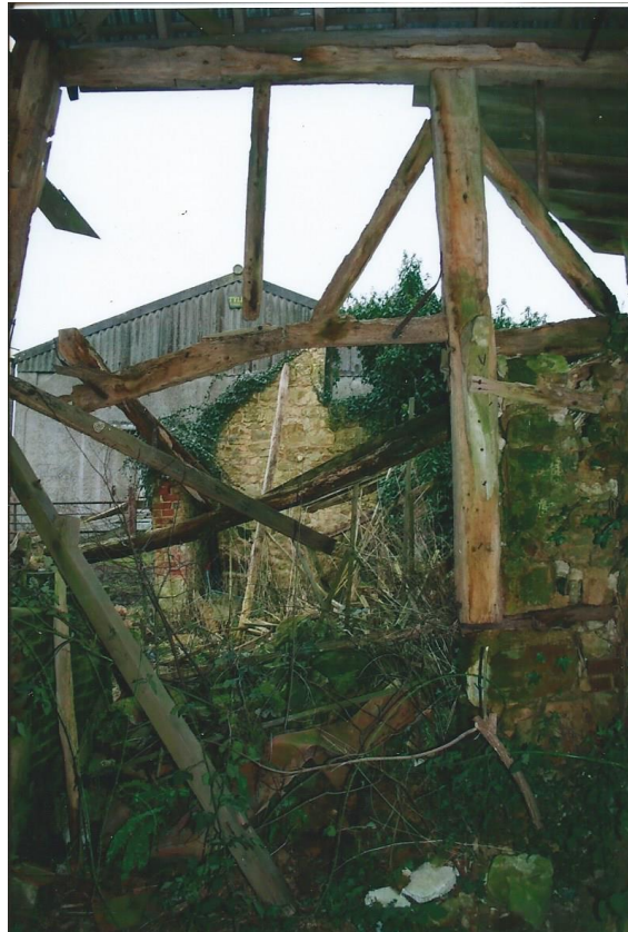
Plate 25 Before client renovating the south east corner (Reproduced by kind permission of Jamie French)
