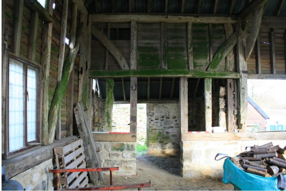
Plate 10. The north elevation between truss A and B with outshot beyond (scales 1m and 50cm)
