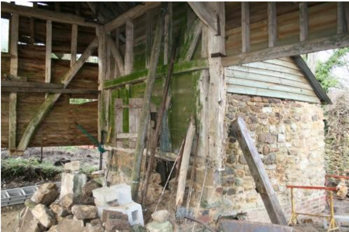
Plate 31 During renovating inside looking north west (Reproduced by kind permission of Jamie French)
