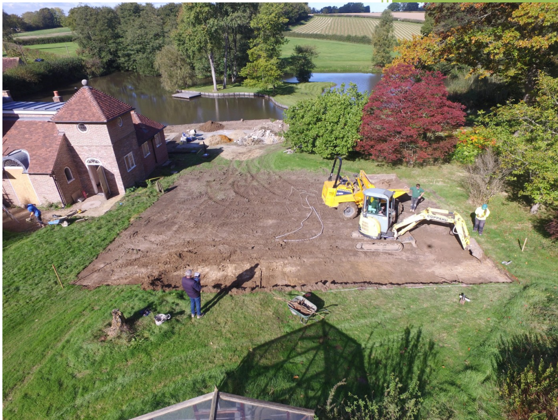
The excavation of Area 1 in progress with the top of [102] and [105] exposed.
