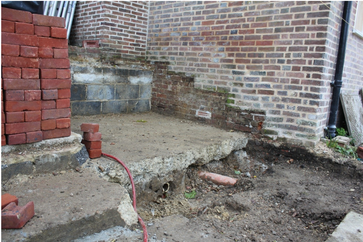
Plate 1. Area 3 showing removal of block and beam steps on top of thick concrete.
